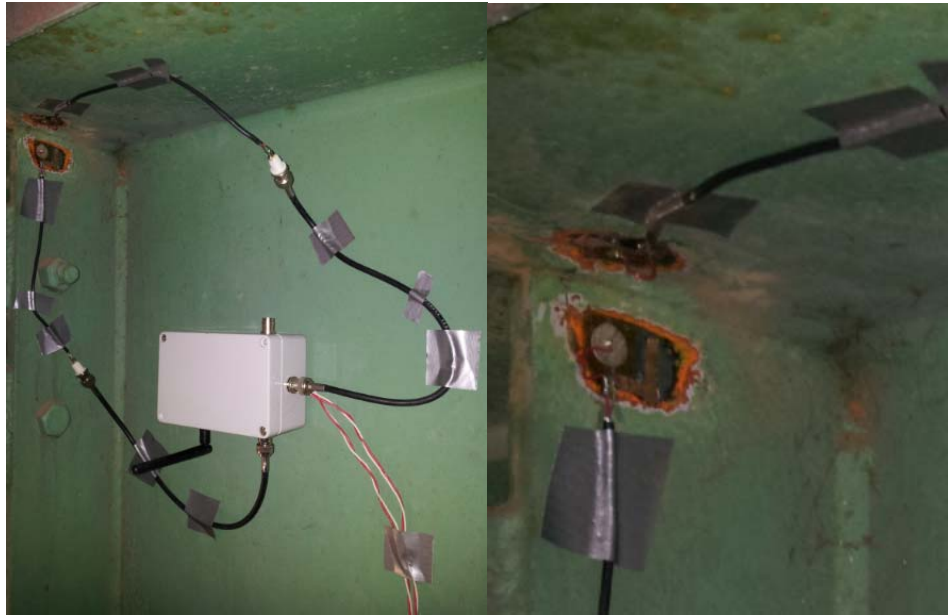
Figure 12 - Wireless AE Sensor (Left) and Crack (Right)
