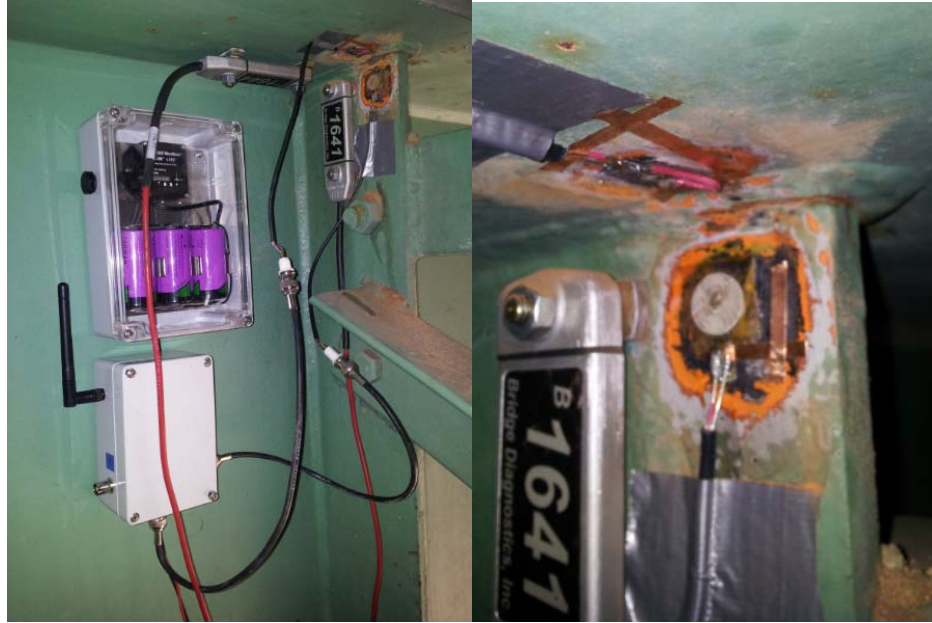
Figure 11 - Wireless AE Sensor (Left) and Crack (Right)
