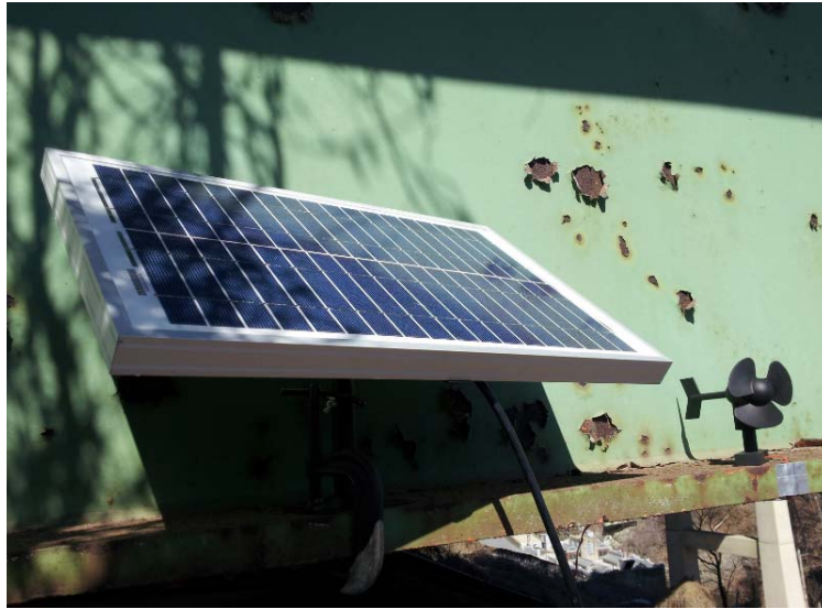
Figure 13 - Solar Panel (Left) and Wind Turbine (Right)
