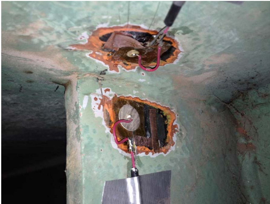
Figure 5 - Piezo film AE sensors installed on Girder #2 of I-95 Bridge to monitor existing fatigue crack
