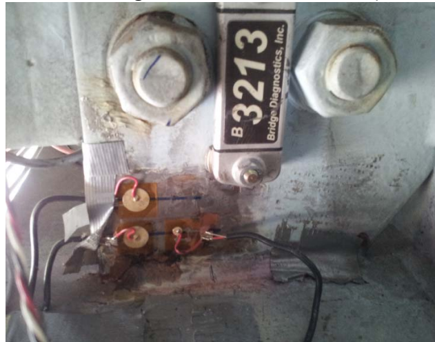
Figure 18 Piezo Film Sensors and PZT Sensor on the Bridge Deck (Piezo Film Sensors: Left Two, PZT Sensor: Right One)
