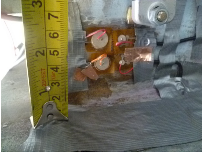
Figure 3. New installation of piezoelectric film AE sensor near existing fatigue crack on connection plate on Girder #3
