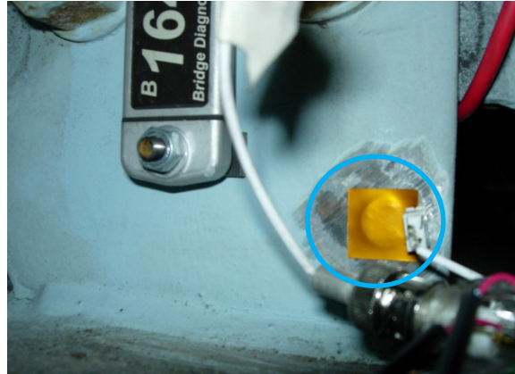
Figure 9. Piezoelectric paint AE sensor (blue circled, for monitoring ambient noise since there is no fatigue crack on this side connection plate)
