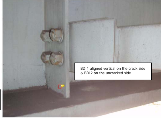
Figure 5. No Sign of Cracking at G3B3D3 (Girder 3 Bay 3 Diaphragm 3) and one
