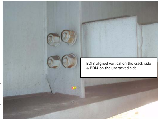
Figure 7. No Sign of Cracking at G4B4D3 (Girder 3 Bay 4 Diaphragm 3) and one sensor
