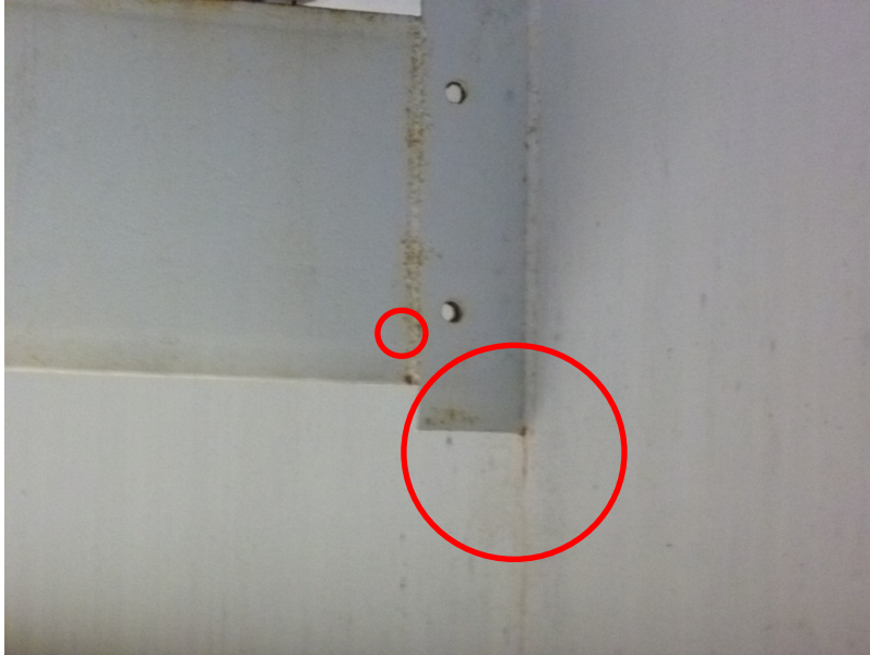
Figure 3. Fatigue crack on girder web location (at the weld intersection of diaphragm and web plate)
