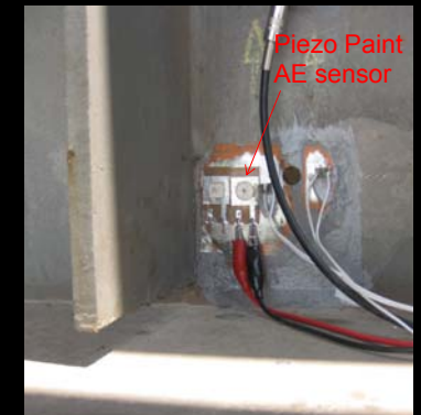
Existing fatigue crack
